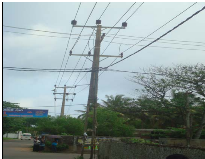
Figure 2.3 Photograph of Ratmalana Feeder - 9
