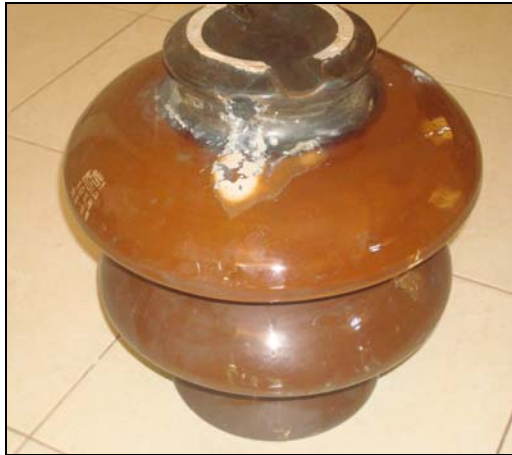
Figure 2.4 The Flashover 33kV Pin Insulator
