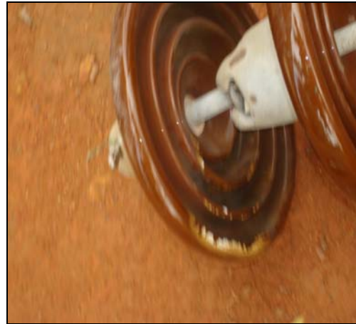
Figure 2.5 The Flashover 33kV Shackle Insulators
