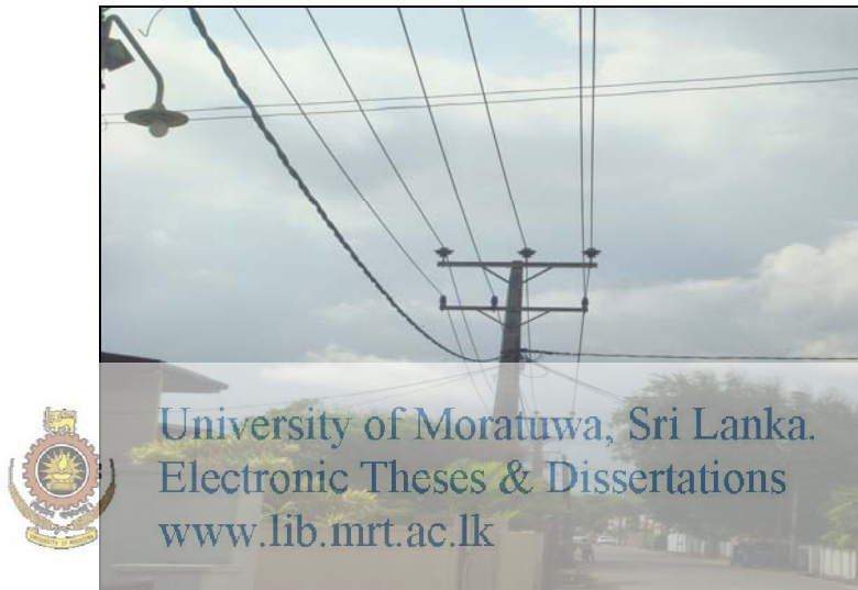
Figure 2.2 Photograph of Ratmalana Feeder - 9
