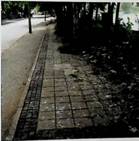
Fig. 4.12 The crows and bats dirty on the road. Credit: Gunasinghe W.K.D.
