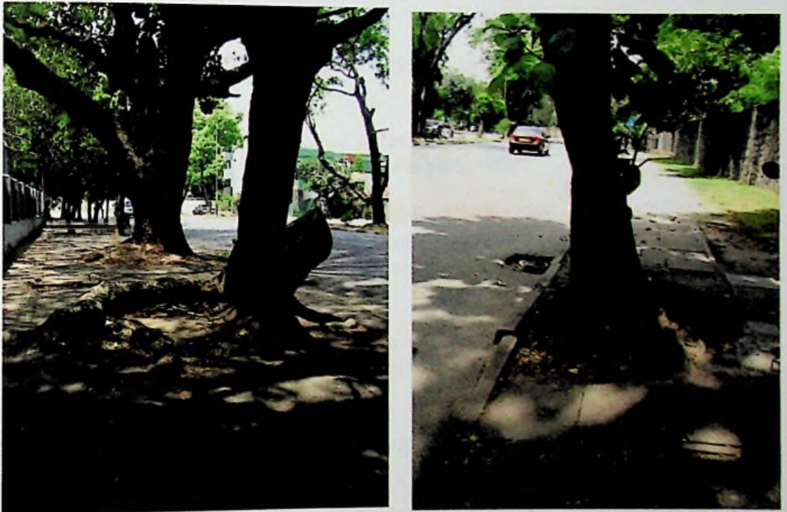
Fig.3.16 The Samanea saman trees and Turmanalia cattapa tree root system come over the surface damage the pavement and cause difficulties for pedestrians.
