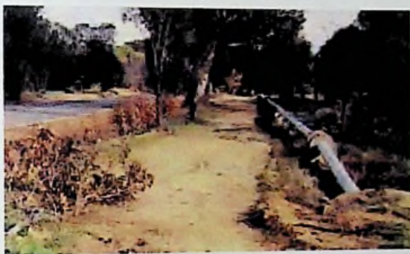
Fig. 6.7. Pipelines form a continuous disturbance along roadsides.
