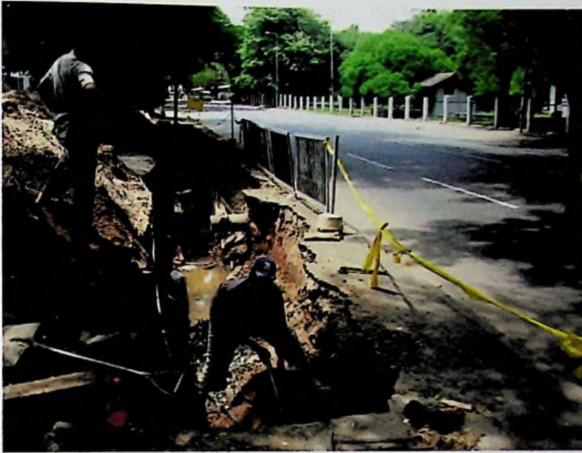
Fig. 3.11 Ceylon Electricity Board, Sri Lanka Telecommunication and Water and Drainage board labourers working at the roadside. This work frequently damages tree roots, weakening trees and making them vulnerable to wind throw during high wind and storms. Credit: Gunasinghe W.K.D.
