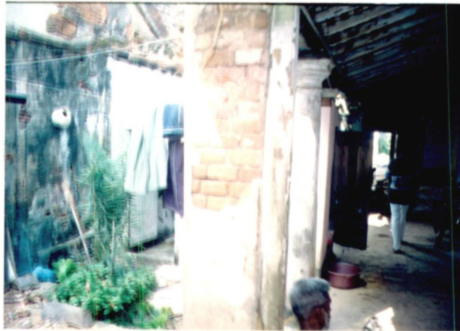
Part of open court adapted to function as common toilets and showers
