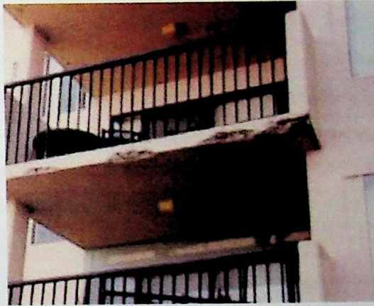
Figure 3.2: Spalling of concrete
