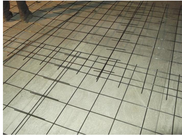
Figure 2: Reinforcement net on a pre-stressed concrete slab panel before prior to screed concreting
