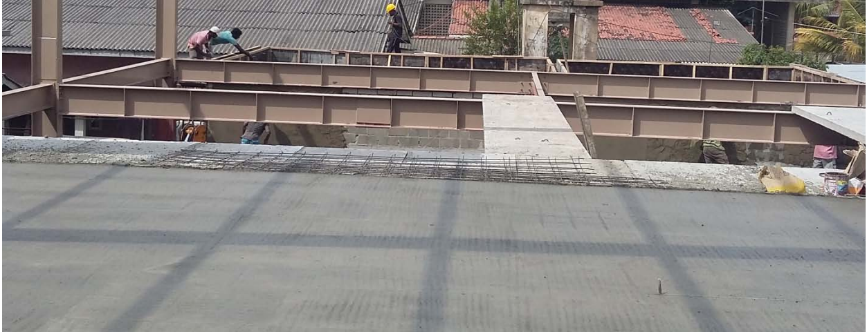
Figure 7: Pre-cast Pre-tensioned slabs spanning on steel beams with a reinforced in-situ topping on top
