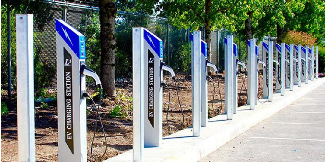
Figure 3:4: Portland Airport Level 1 charging station [37]
