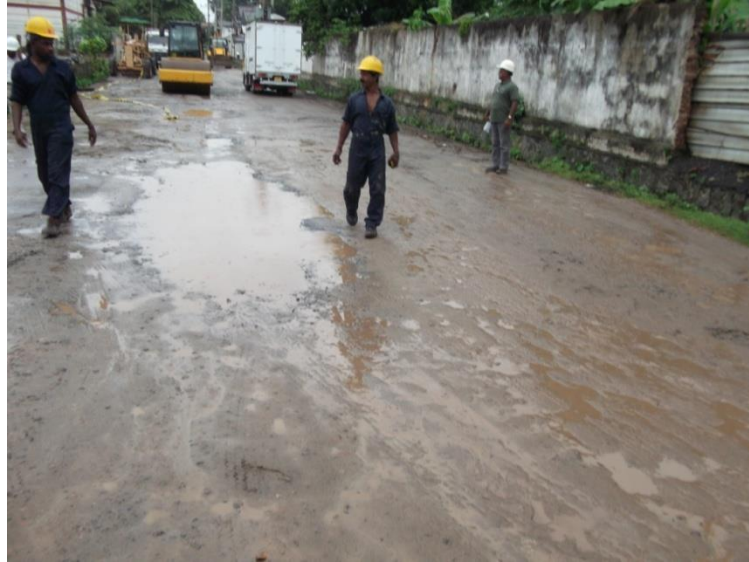
Figure 4.5: Muddy and unleavened road surfaces just after completed work of New Airport road
