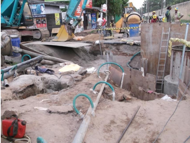
Figure 2.3: Pictures of Settlement of the Ground due to Soil Migration at Deep Trenching at Katukurunduwatta road
