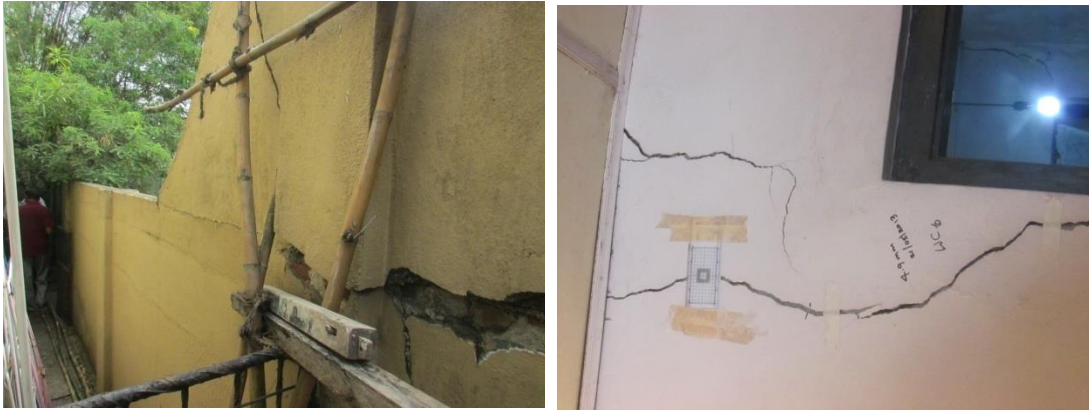
Figure 2.1: Pictures of Damaged houses at KandawalaMawatha
