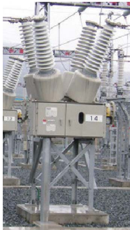
Figure 5.8 - Medium Voltage Circuit Breakers
