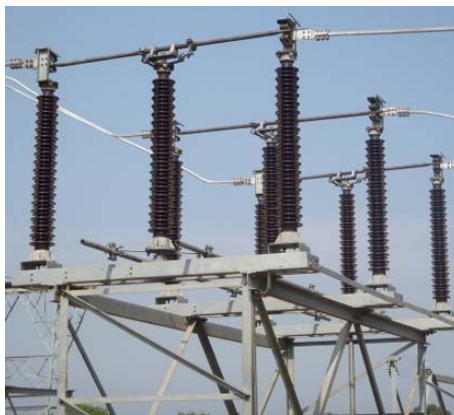
Figure 5.6 - High Voltage Isolator
