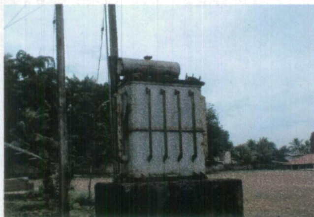
Figure 4.3 A decommissioned transformer
