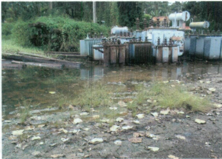
Figure 4.4 Unsound practices of storage of decommissioned transformers
