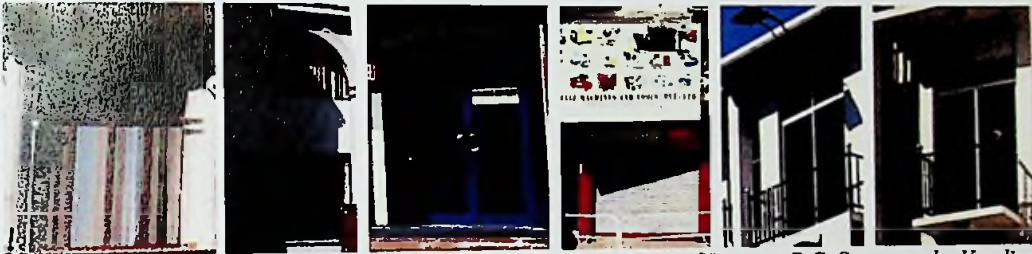
Fig.139 Altered Windows designs with new materials and colour of Present D.S. Senanayake Veediya Source. Author
