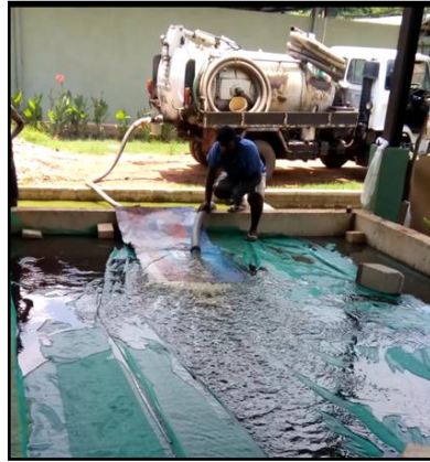
Figure 14 - FS discharge in to the sand beds
