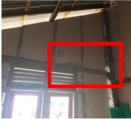
Figure 4-16: Inside of the model House Same location; inside view; Red color area was captured by thermal camera.
