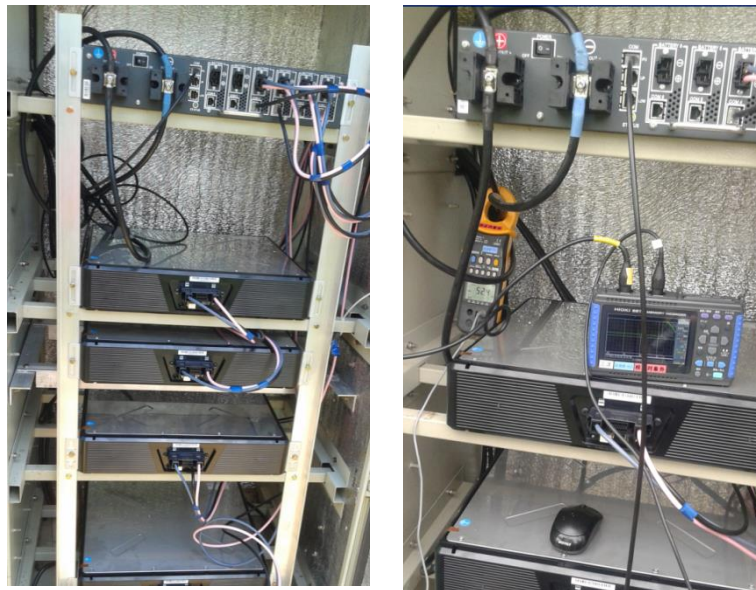
Figure 7.7 : Tested Li Ion 300Ah Battery Bank at Karandana Mobitel Site
