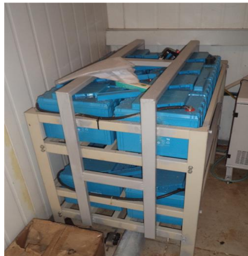
Figure 7.2 : Installed 800Ah Fiamm VRLA Batter Bank at Welimuwapotana Dialog Site
