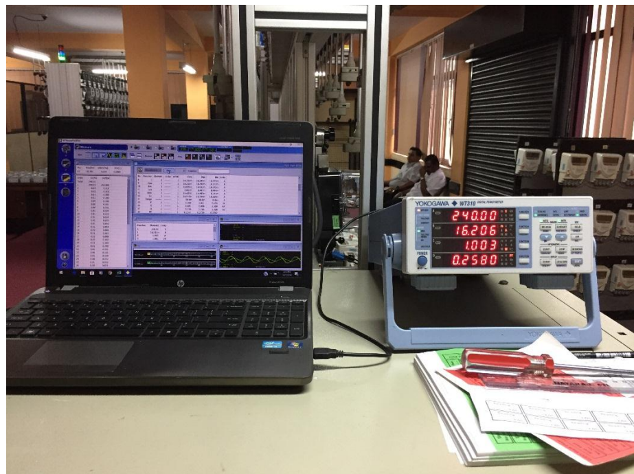
Figure 3-15 Image 2 of testing Power Consumption of Electromechanical Meter
