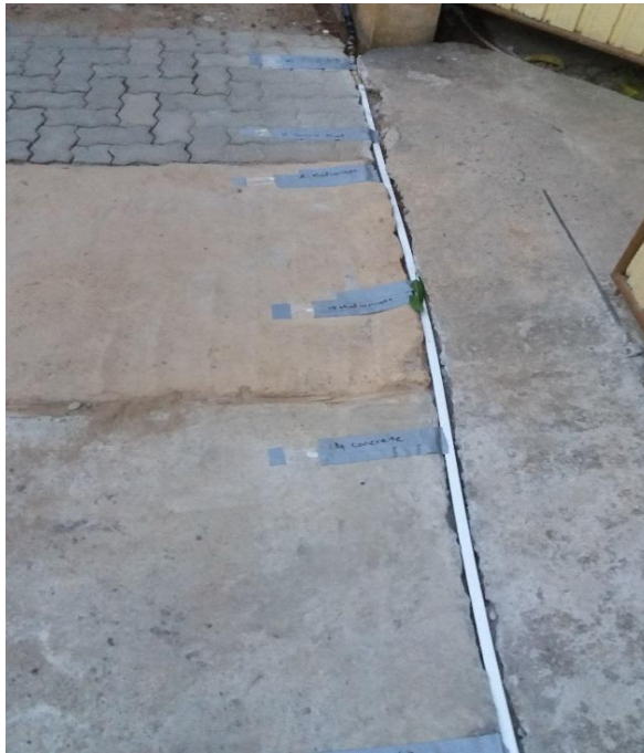
Figure 29- Sensors attached on surface of each material
