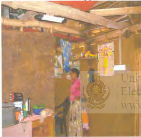
Wiring on Roof Rafters & Light
