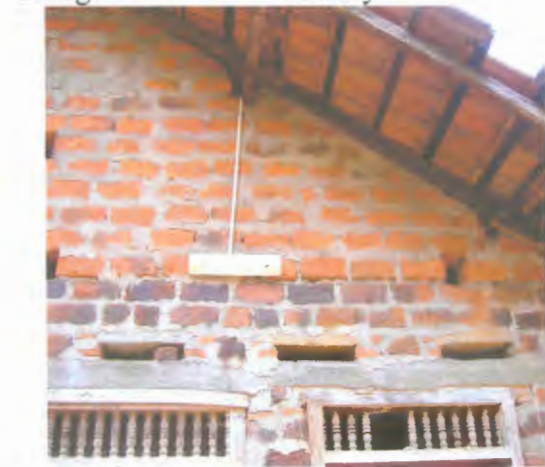
DC Light – Florescent
