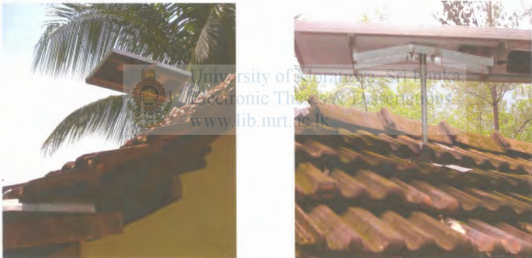
Figure 4.2.1: Pictures Depicting Module Support Structures
