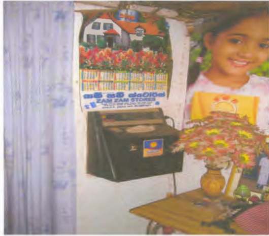
Charge Controller & Battery Box
