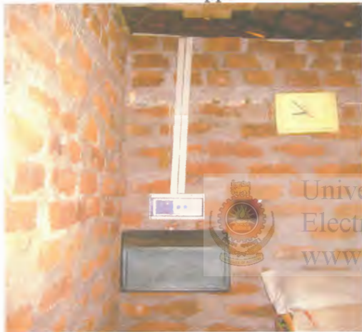
Charge Controller & Battery Box
