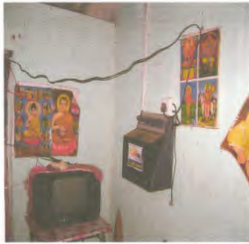
Charge Controller & Battery Box
