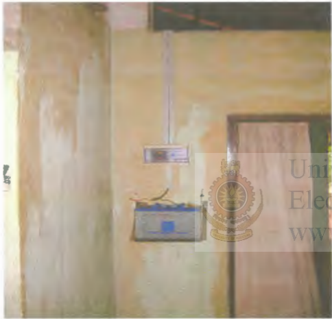
Wiring on Walls Surface
