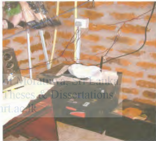
Wiring on Walls Surface
