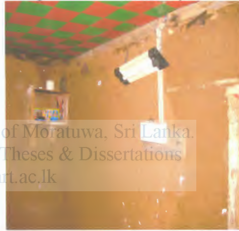
DC Light – Florescent
