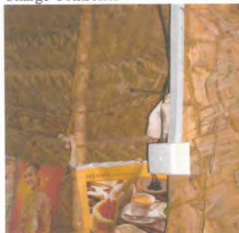
Wiring on Walls Surface
