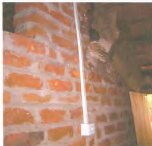
Wiring on Walls Surface
