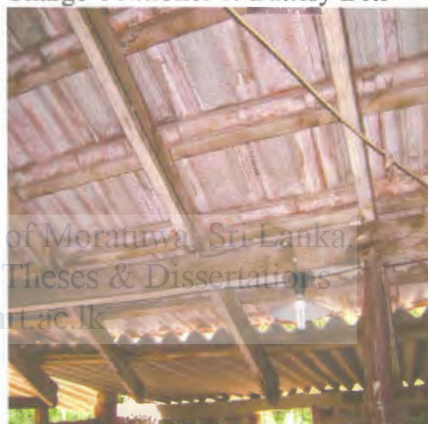
Wiring on Roof Rafters & Light
