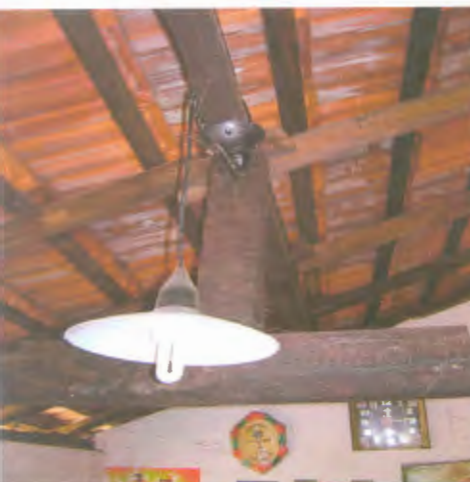
Wiring on Roof Rafters & Light
