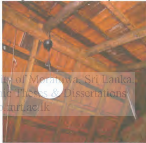
Wiring on Roof Rafters & Light
