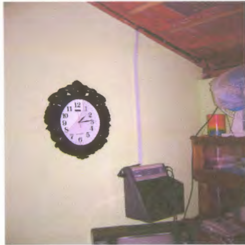
Charge Controller & Battery Box
