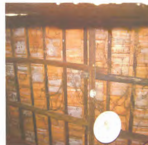
Wiring on Roof Rafters & Light
