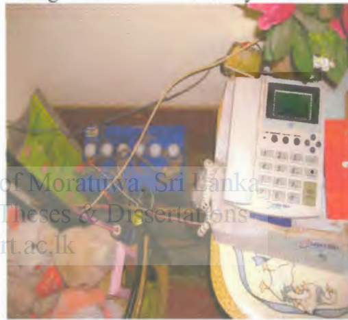
Battery and Box
