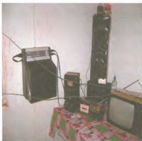
Charge Controller & Battery Box
