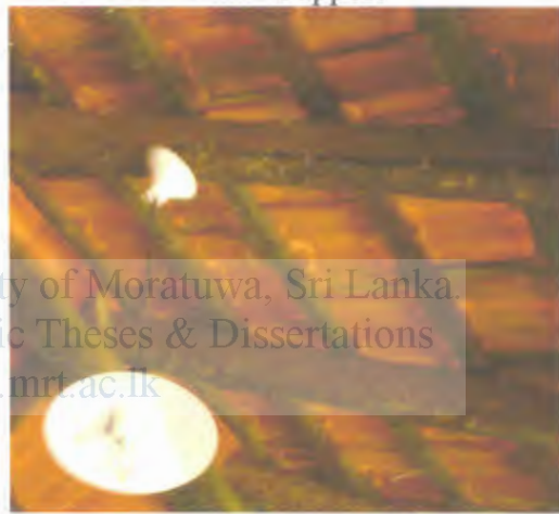
Wiring on Roof Rafters & Light
