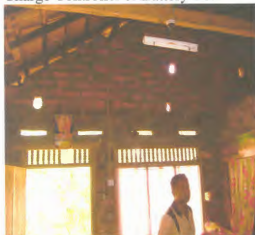
Wiring on Walls Surface & Loads
