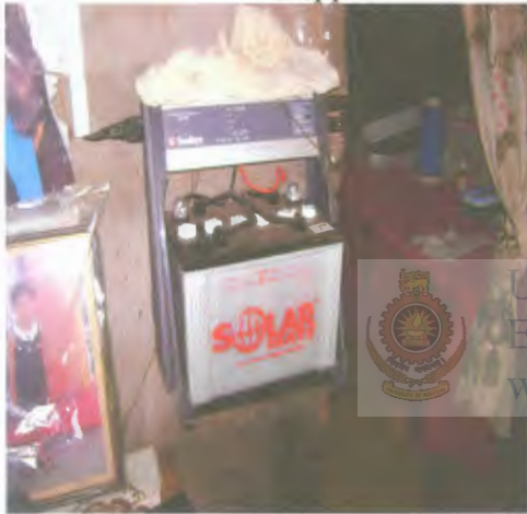
Charge Controller & Battery
