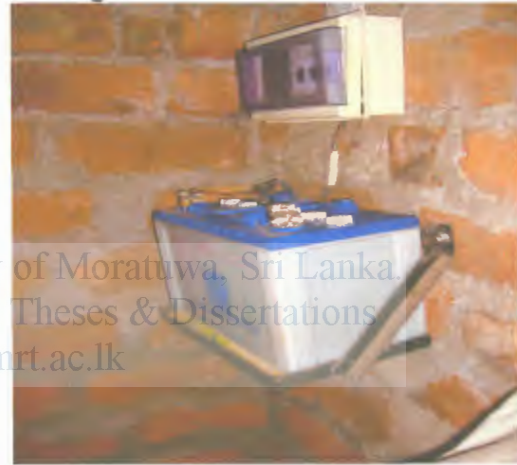
Charge Controller & Battery
