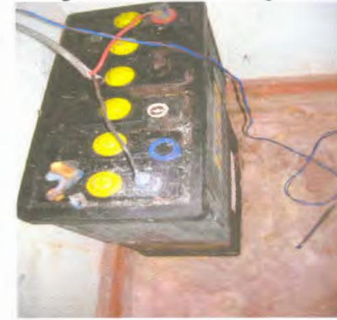
Deep Cycle Solar Battery
