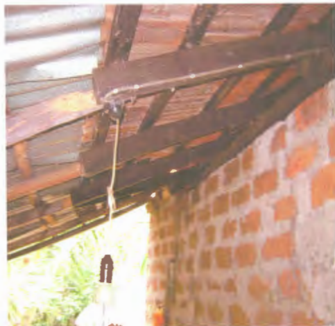
Wiring on Roof Rafters & Light
