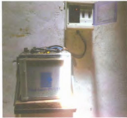
Charge Controller & Battery
