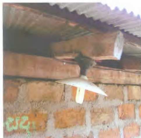
Wiring on Roof Rafters & Light
