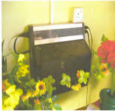
Charge Controller & Battery Box
