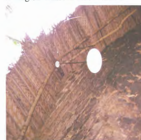
Wiring on Roof Rafters & Light
