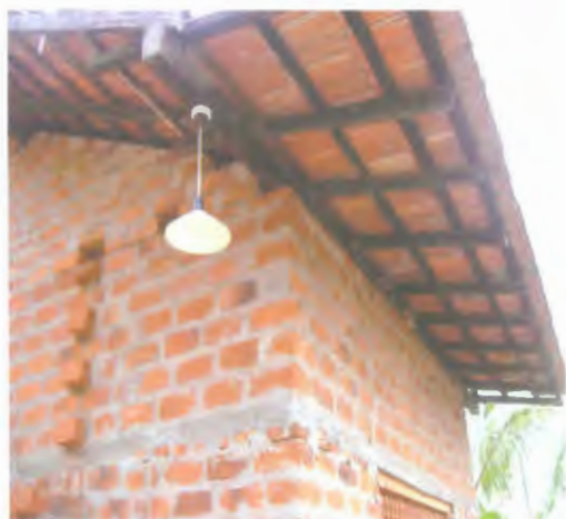
Wiring on Roof Rafters & Light
