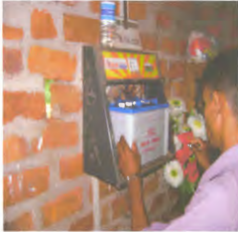
Charge Controller & Battery
