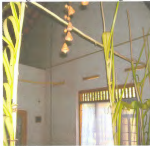
Wiring on Walls Surface
