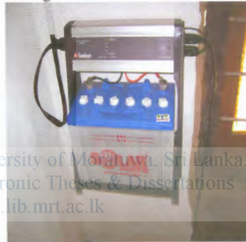
Charge Controller & Battery
