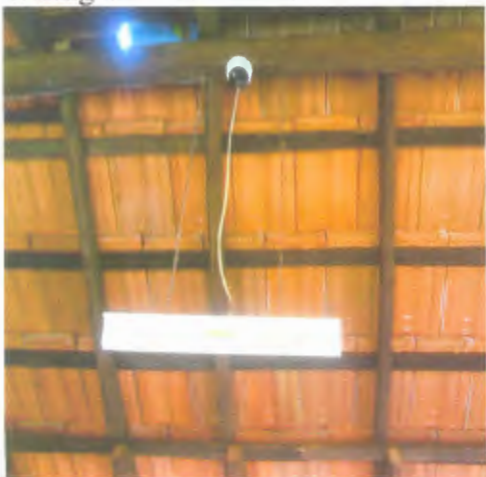
Wiring on Roof Rafters & Light
