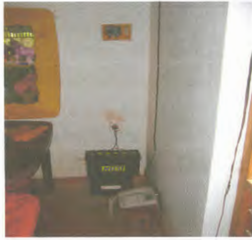
Charge Controller & Battery
