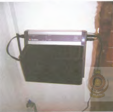
Charge Controller & Battery Box
