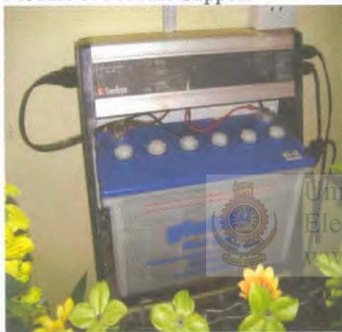
Charge Controller & Battery
