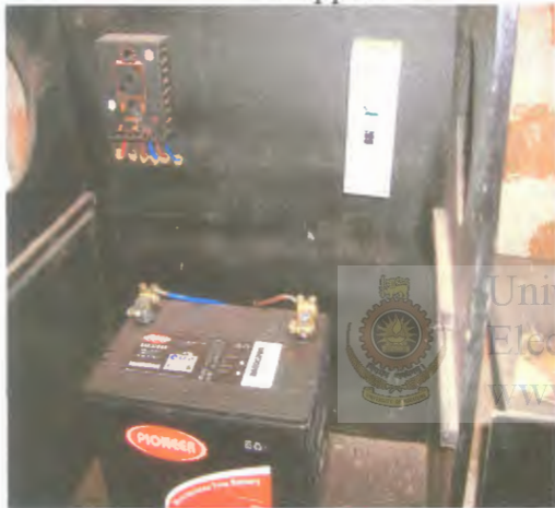
Charge Controller & Battery
