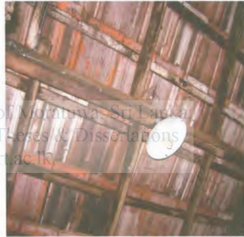
Wiring on Roof Rafters & Light
