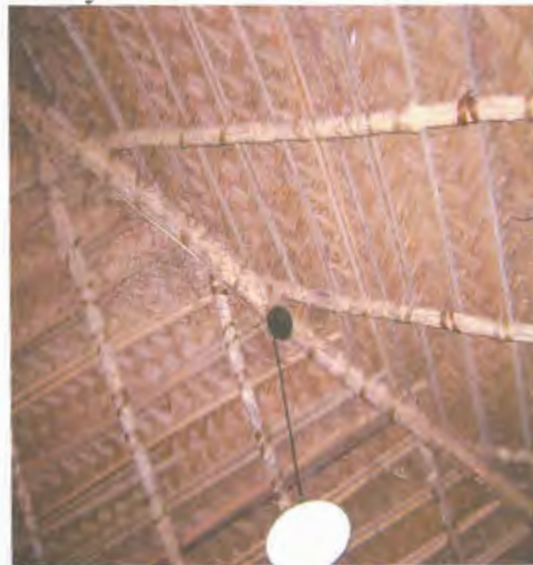
Wiring on Roof Rafters & Light
