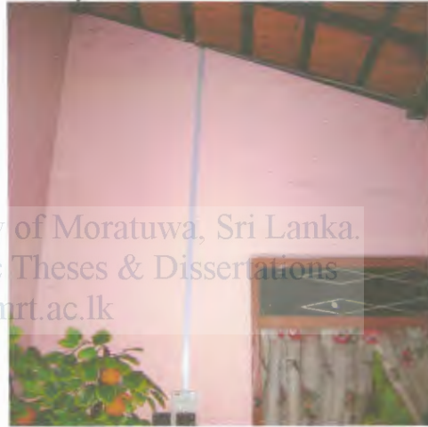
Wiring on Walls Surface
