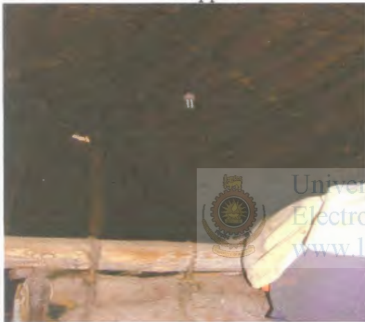
Wiring on Roof Rafters & Light
