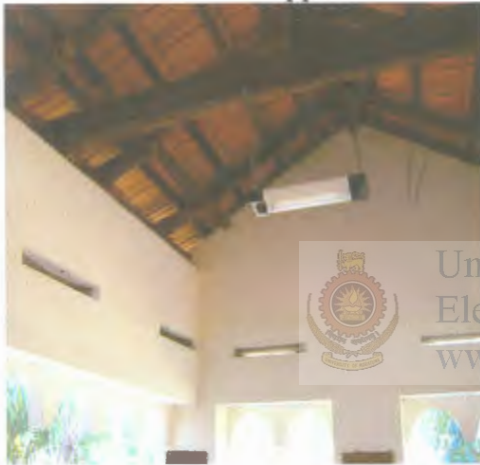
Wiring on Roof Rafters & Light
