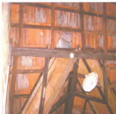
Wiring on Roof Rafters & Light
