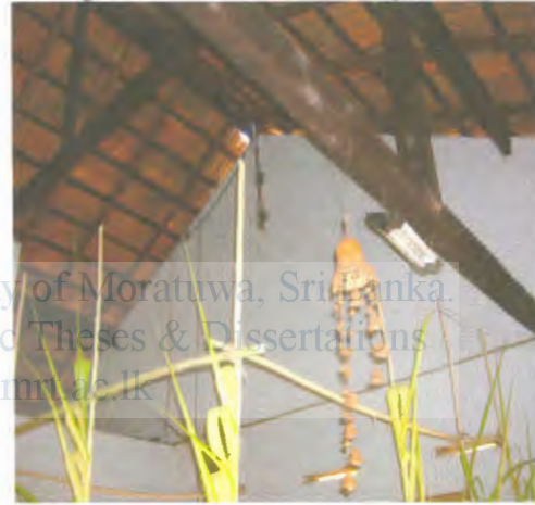
Wiring on Roof Rafters & Light
