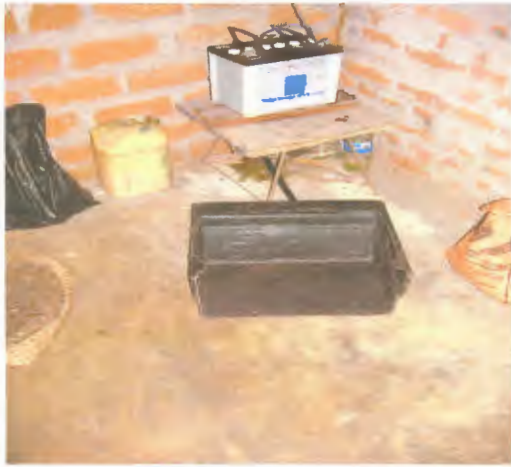
Charge Controller, Battery & Battery Box
