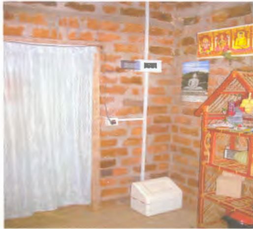
Charge Controller & Battery Box
