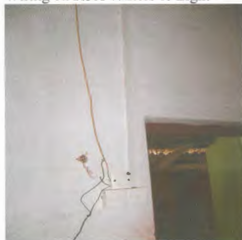
Wiring on Walls Surface
