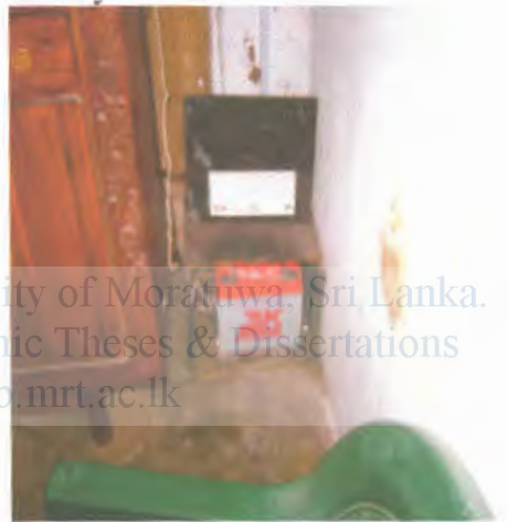
Battery and Box
