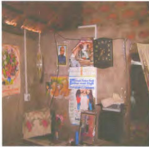
Charge Controller & Battery Box
