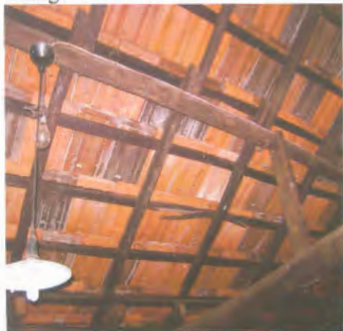
Wiring on Roof Rafters & Light
