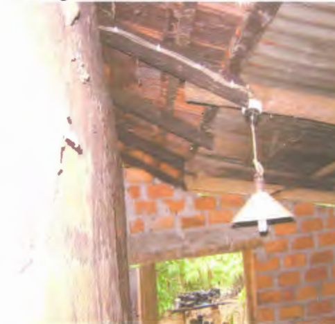
Wiring on Roof Rafters & Light
