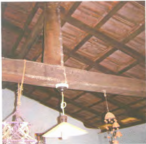
Wiring on Roof Rafters & Light
