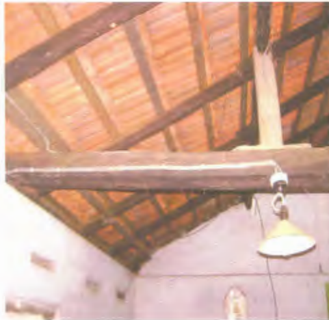
Wiring on Roof Rafters & Light
