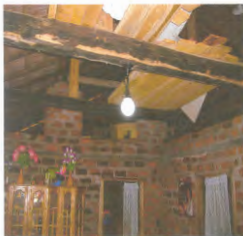
Wiring on Roof Rafters & Light
