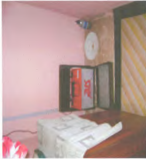
Battery and Box
