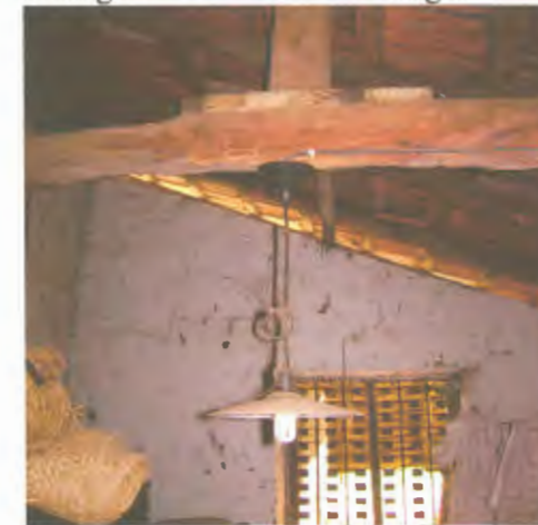
Wiring on Roof Rafters & Light
