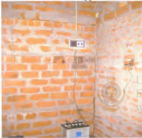
Wiring on Walls Surface
