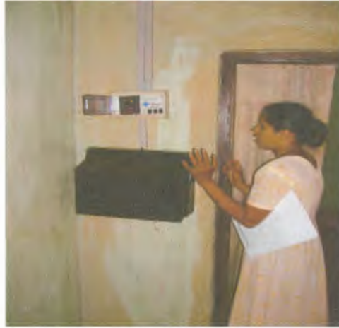
Charge Controller & Battery Box
