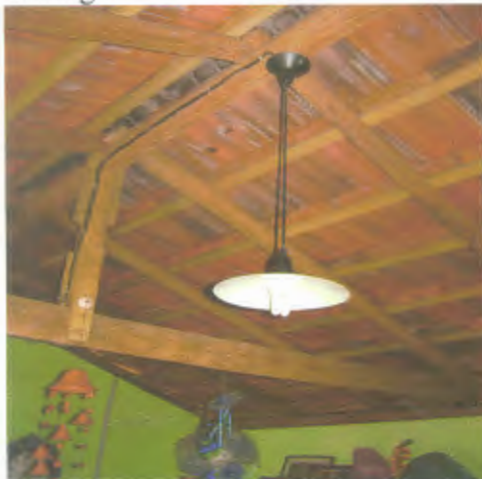
Wiring on Roof Rafters & Light
