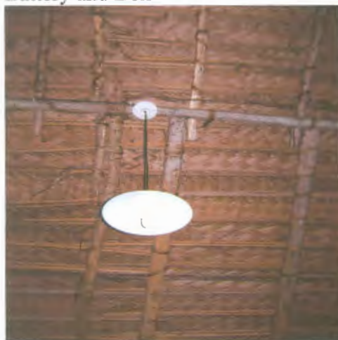
Wiring on Roof Rafters & Light
