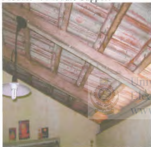
Wiring on Roof Rafters & Light
