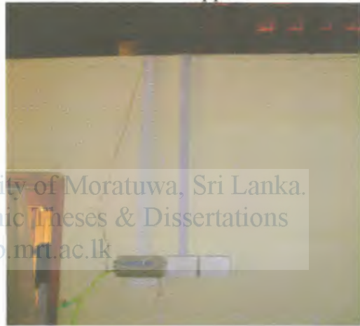
Wiring on Walls Surface
