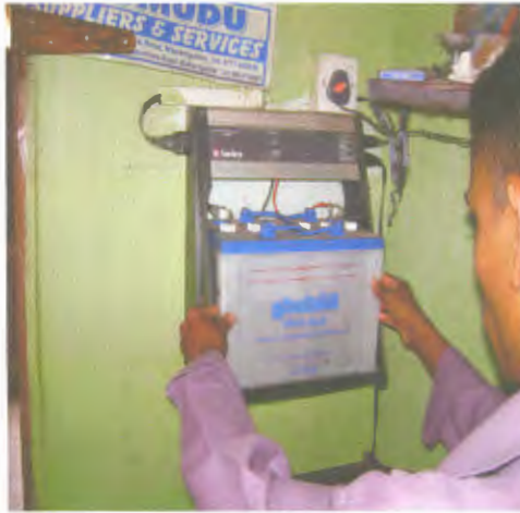
Charge Controller & Battery
