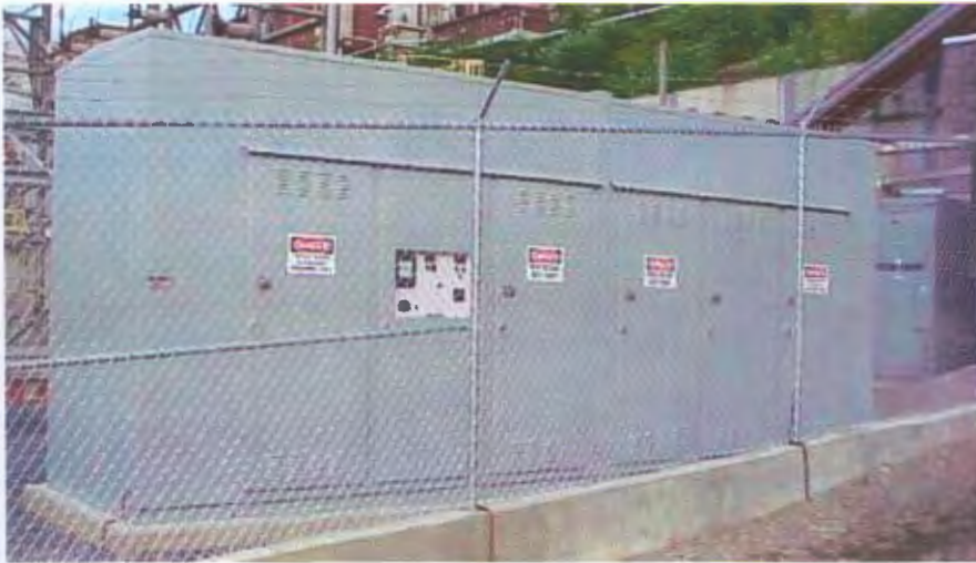
Figure 3.2 Typical pad mounted Capacitor bank
