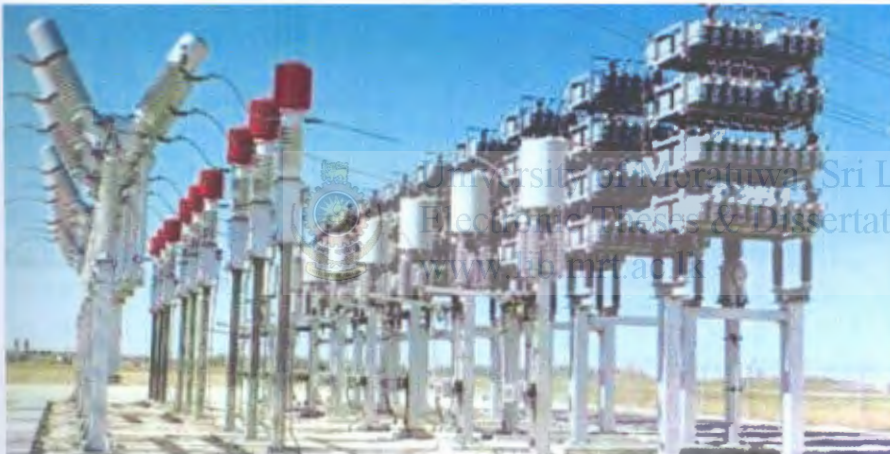
Figure 3.3 Stacked rack capacitor bank
