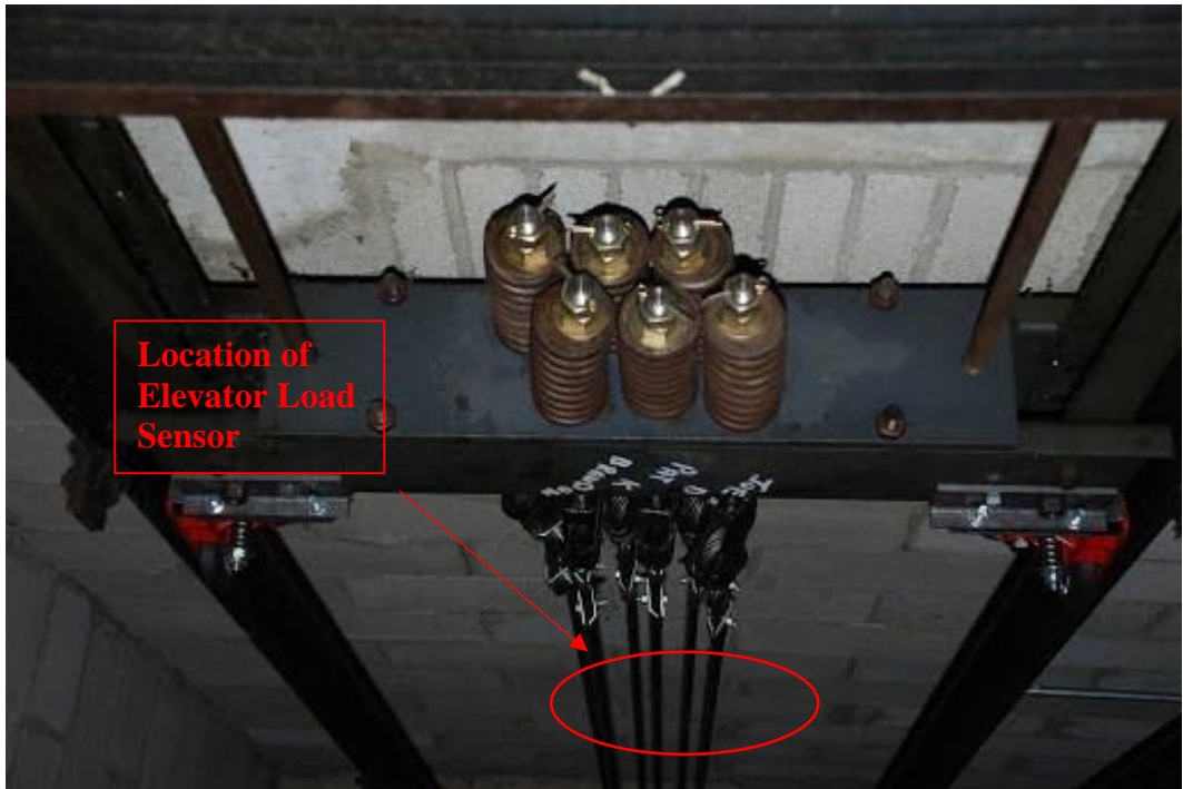
Figure 3.8: Mounting location of elevator load sensor
