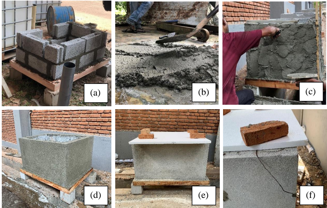
Figure 98. Building prototype (a) Construction of building prototype; (b) preparation of mortar mix; (c) External plaster application; (d) Completed prototype; (e) Placing EPS roof panel (f) Monitoring wall temperature
