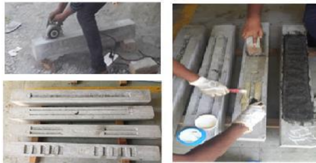
Figure 10: (a) Groove Cutting (b) Filling Grooves with Epoxy and Fixing CFRP Sheets
