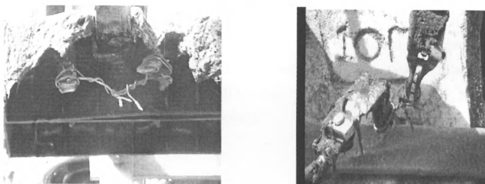
Fig.5.3: Improper electrical connections
