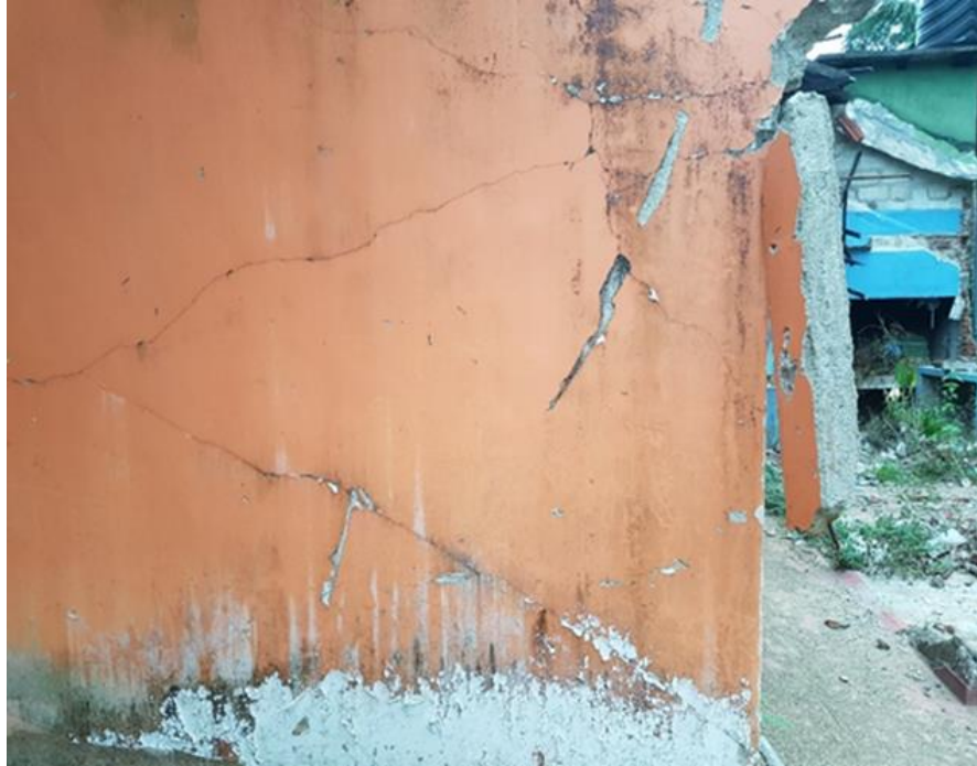
Figure 3. 18: Wall failed in flexure parallel to bed joint
