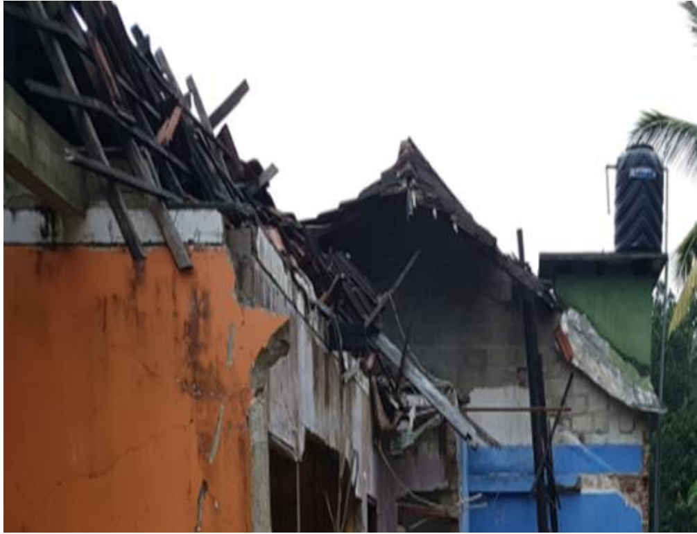
Figure 3. 20: Damages took place in the roof
