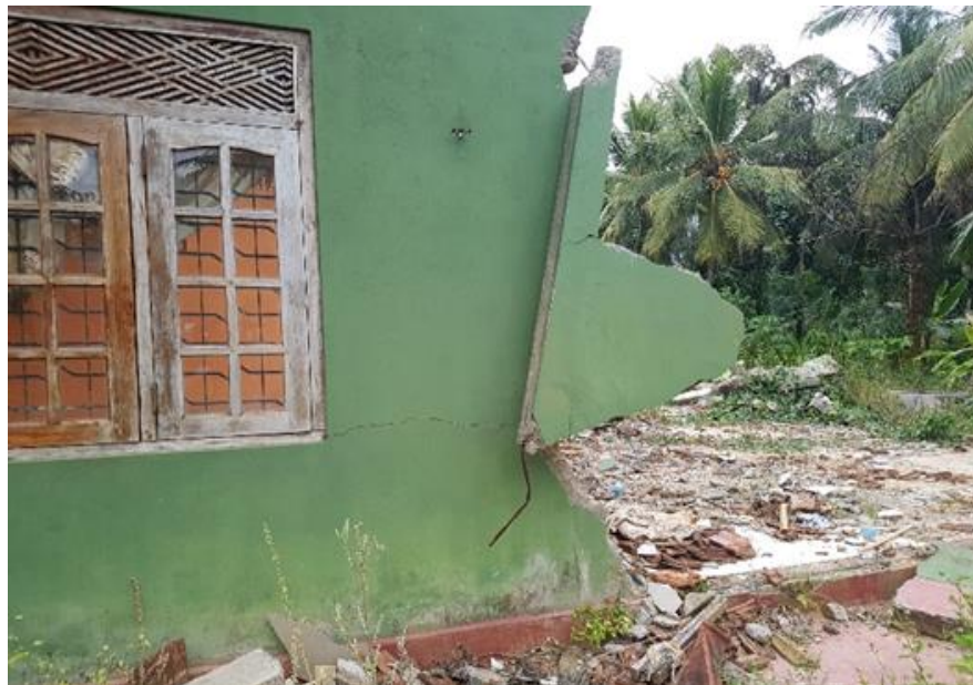
Figure 3. 19: A collapsed and cracked wall
