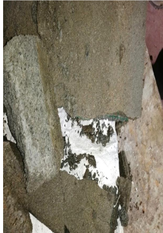
Wire mesh was broken
