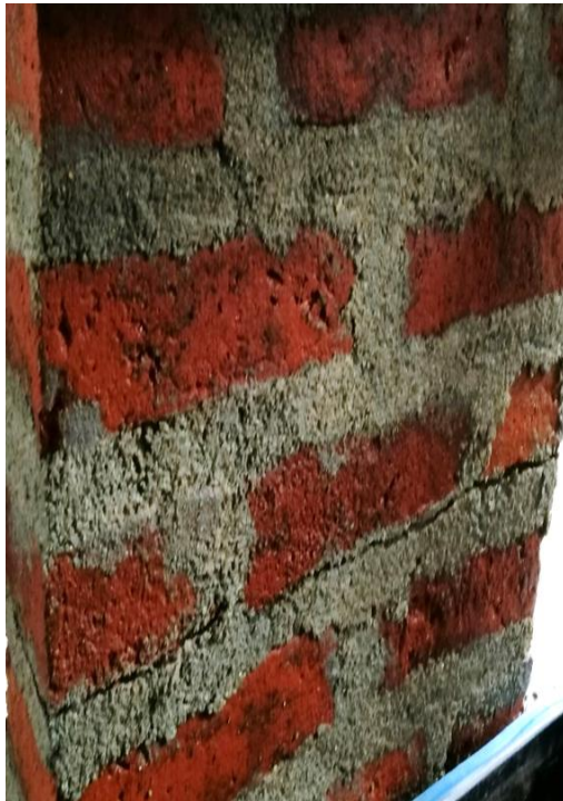
Crack along the bed joint
