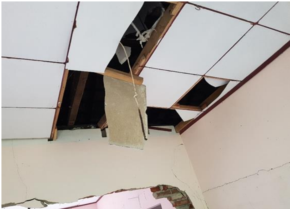
Figure 3. 21: Damages occurred to the plaster board ceilings
