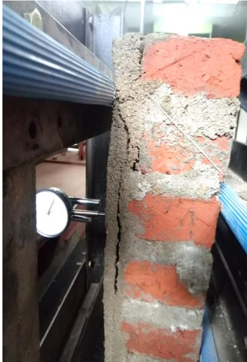
Separation of retrofitting material and external plaster
