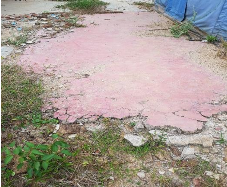
Figure 3. 22: Damages emerged to the floor
