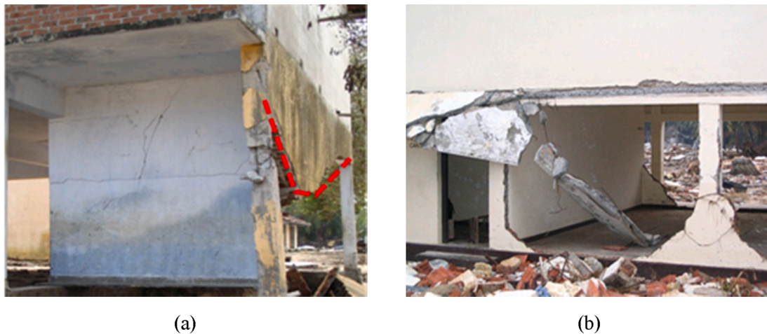
Fig. 8. Out of plane failure modes observed in infill walls of school buildings in Sri Lanka under the 2004 Tsunami: (a) tsunami mainly acting along the x direction, and (b) tsunami mainly acting along the y direction.
