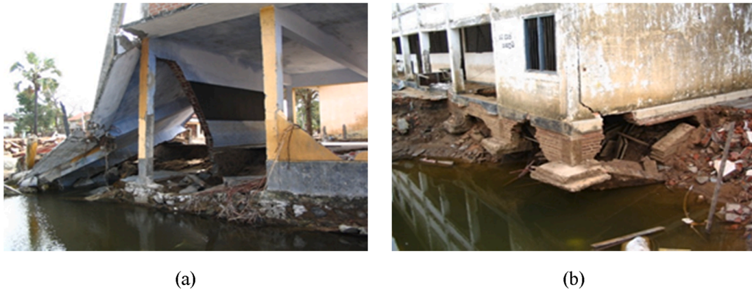
Fig. 6. Damage after the 2004 tsunami on existing schools caused by the scour.
