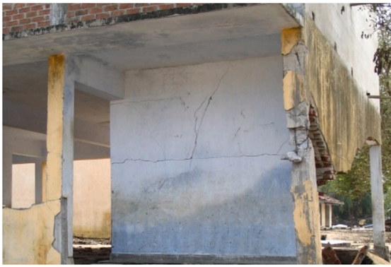
Fig. 12. Shear failure observed in a corner column of a typical school building after the 2004 tsunami.
