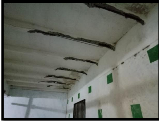
Figure 3.10: Deterioration of NERD slab system
