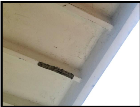
Figure 3.12: Deterioration of Pre-stressed NERD slab purlins in house located in Ekala
