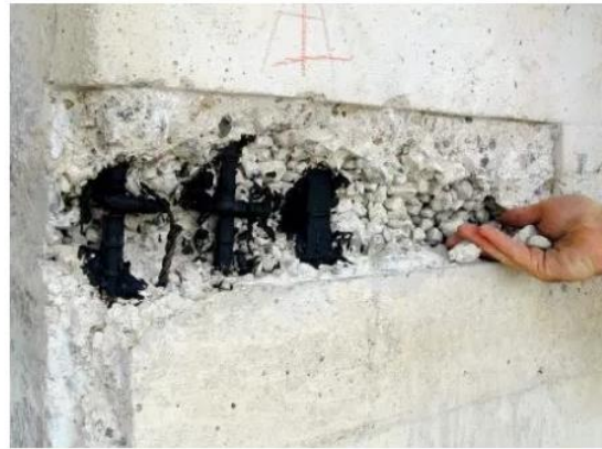
Figure 2.10: Remove damaged concrete, cut spalling concrete, brush steel bars, and coat steel bars (the constructor)
