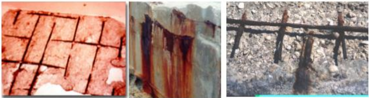
Figure 2.14: Images of several types of rust damage. (When spalling occurred, localized corrosion (center) and overall corrosion owing to carbonation (left, right)) (Ziga Smit, 2008)
