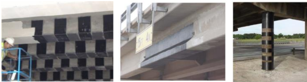
Figure 2.24: Application of CFRP for (a) flexural stiffness (b) shear strengthening (c) axial confinement.
