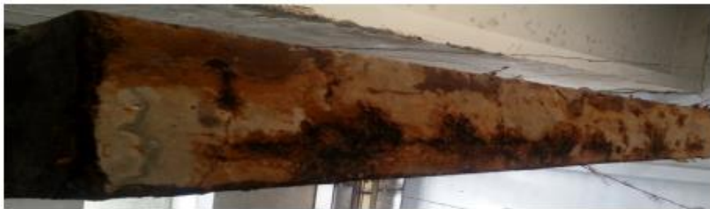
Figure 2.28: the crack pattern of corroded concrete specimen
