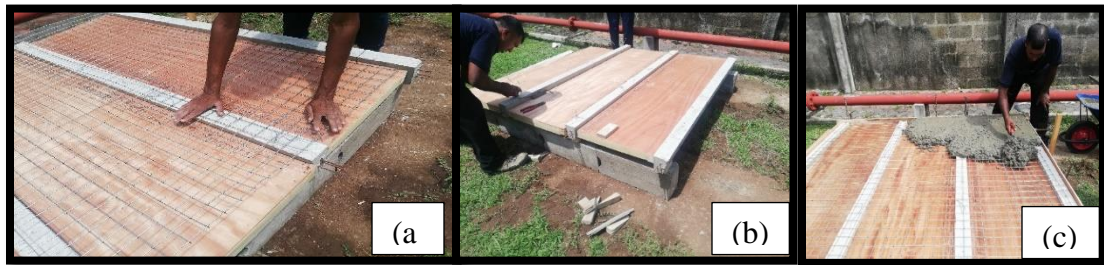
Figure 2.9: Casting the composite slab panel (a) Hang the plywood shutter (b) keeping the welded mesh at the center (c) Making the in-situ topping.
