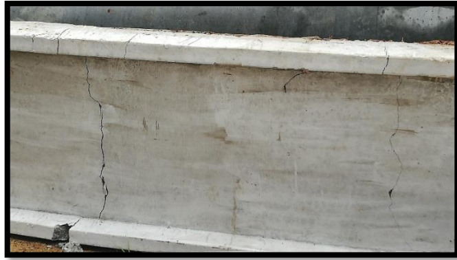
Figure 5.2: Slab failure at two supports
