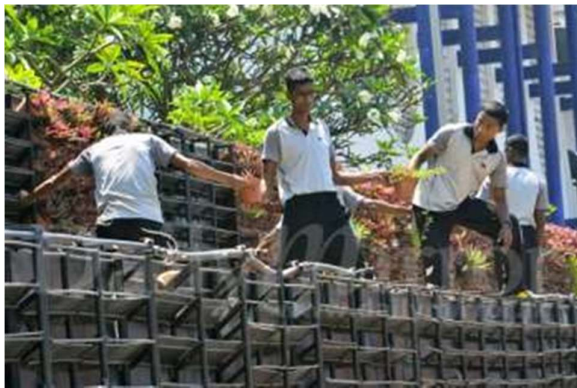
Figure 15. Temple trees boundary wall while removing the green wall Source: Daily Mirror
