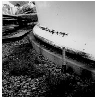
Figure 2-15: Elephant's foot buckling failure of hollow sections (Haroun, 2005)
