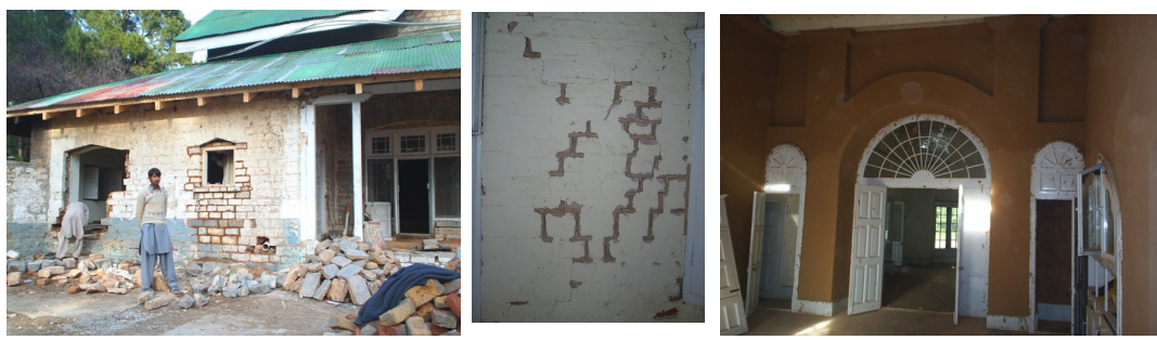
Fig. 12, 13 & 14: Frontier House Inside and Outside View during and after work. Source: Author
