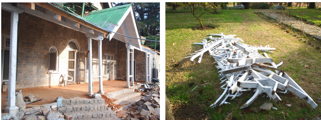
Fig. 15 & 16: Frontier House Back Side View and damaged wooden handrail Source: Author
