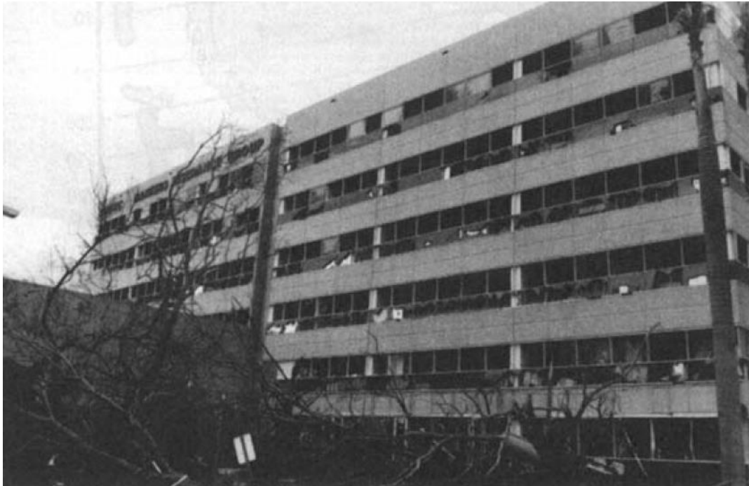
Figure 2.13 - Extensively damaged glass panels of the American Bankers Insurance Group Building, Cutler Ridge, Florida (Behr & Minor, 1994)
