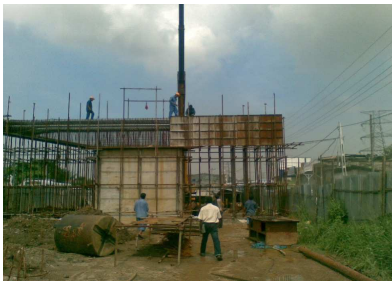
Figure 5 A cantilever of 5.5 m with post tensioning ducts in the pier capping beam
