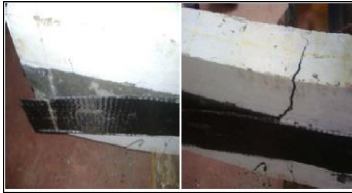
Figure 14: Debonding failure of FRP strengthened slabs
