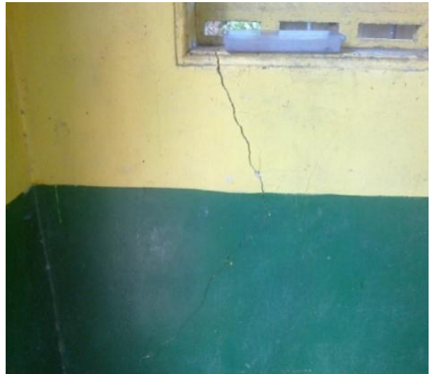
Figure 4 -damage to wall due to tree roots.
