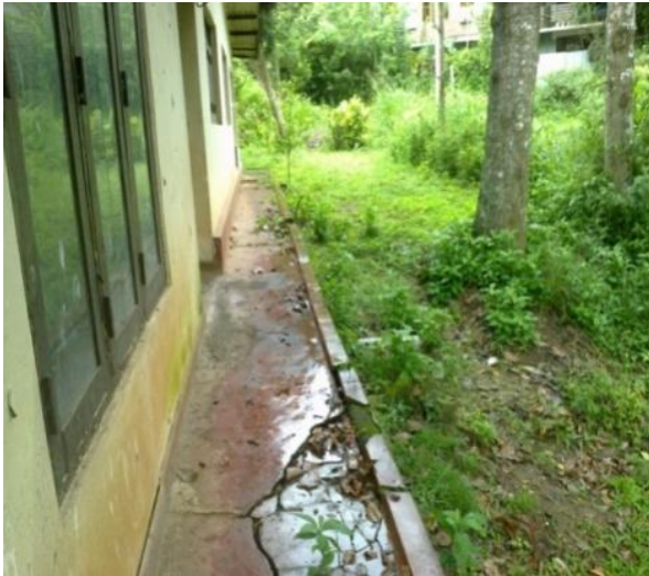
Figure 1 -damage to pavement due to tree roots.
