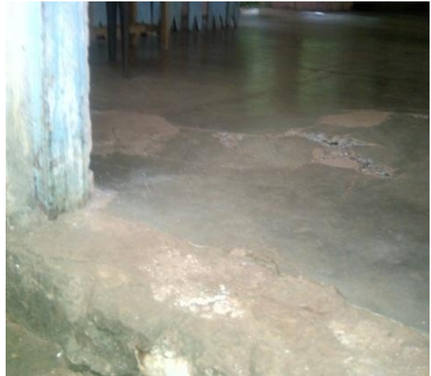
Figure 2 -damage to floor due to tree roots.
