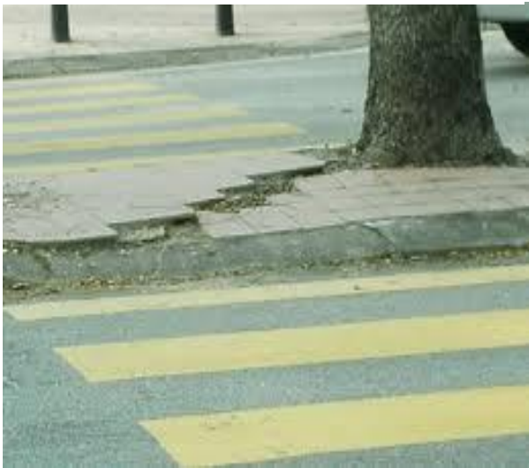
Figure 3 -damage to road due to tree roots.
