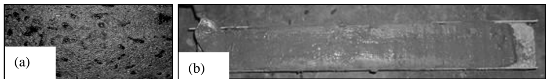
Figure1: (a) Sandblasted surface before applying CFRP sheets, (b) Cement grout layer as adhesive, (c) Applying CFRP layer to the beam
