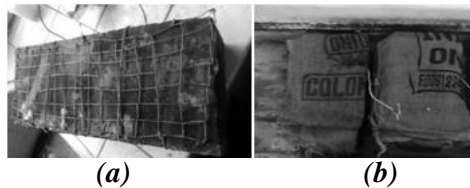
Figure 4: Cathodic protection treatment procedure (a) Copper mesh was fixed (b) Wet sags were laid on the beams
