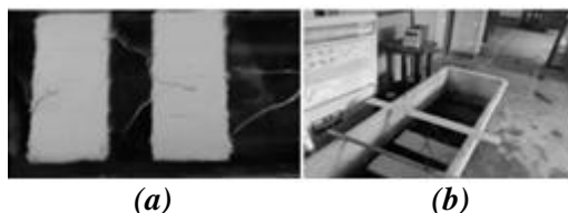
Figure 5: Electrochemical chloride ion extraction treatment (a) \text{Ca(OH)}_2 layer was laid on copper mesh (b) experiment set up
