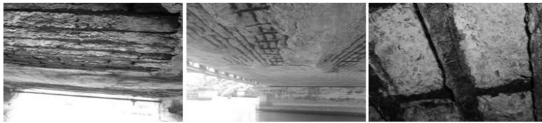
Figure 1: Existing corroded structures
