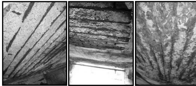
Figure 1: Deteriorated bridge deck slab
