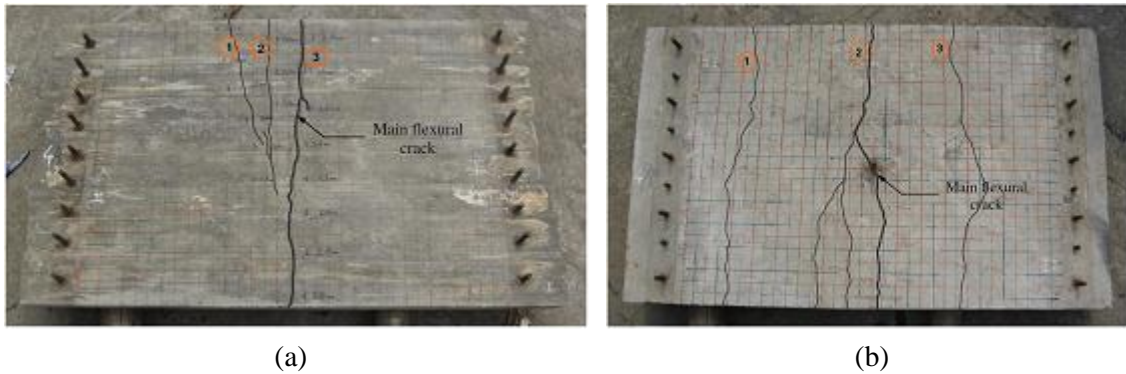
Figure 5: The crack patterns and crack widths on the: (a) top, and (b) bottom surface of specimen UR2
