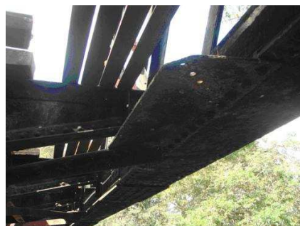
Missing elements and rivets
