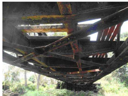
Corroded load carrying elements
