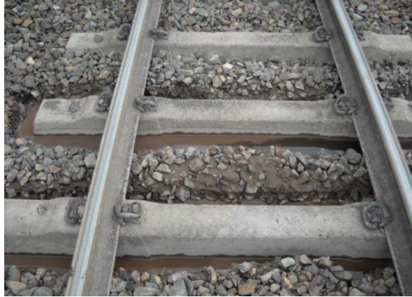
Figure 3: Mudholes caused by excessive coal/clay fouling (Goonyella System, QR National: Photo courtesy of Michael Martin)
