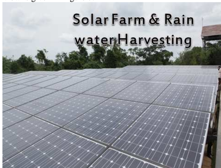
Figure 6: Solar panels arranged to facilitate rain water harvesting
