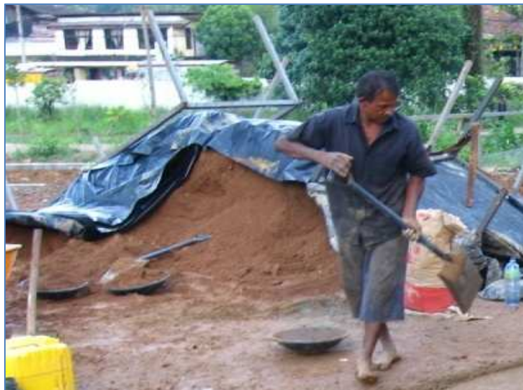
Figure 1: Selected soil is stored with a cover to ensure proper moisture content
