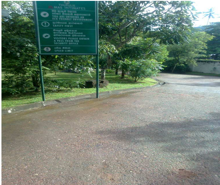
Figure 8: Gradual erosion that has exposed aggregates mixed in wearing course
