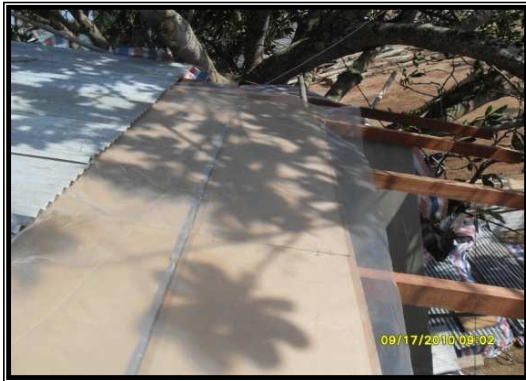
Figure 10: Roof with Dura boards supported on timber joists and also provided with a polythene sheet
