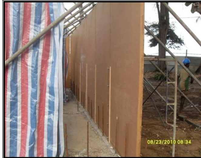
Figure 4: “Dura” Panel wall used for load bearing external walls along with anchors used to connect to the foundation
