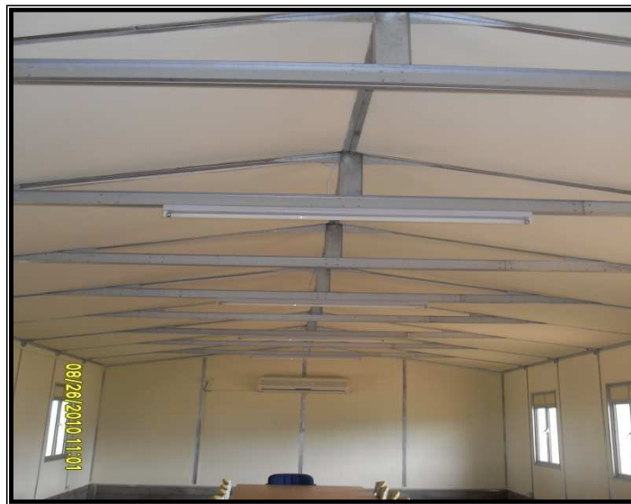
Figure 2: Arrangement of the roof used with Dura as the insulation material and steel members as the truss system.
