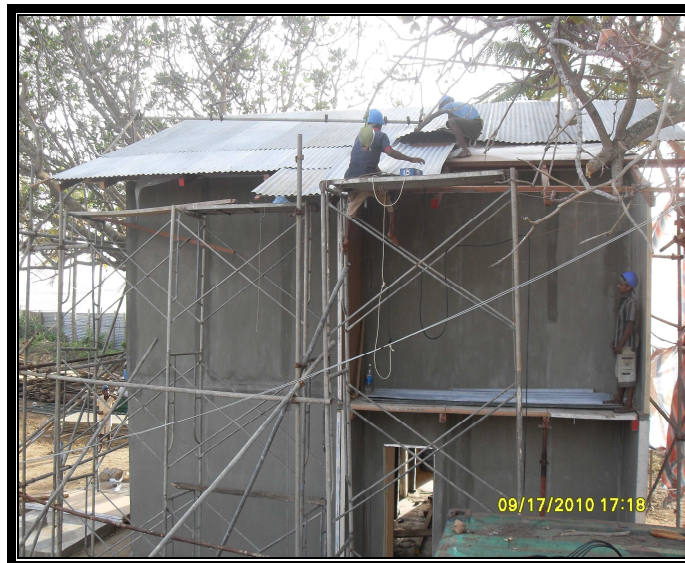
Figure 10: Front elevation of the two storey house under construction at Chaaya Bay hotel at Beruwala
