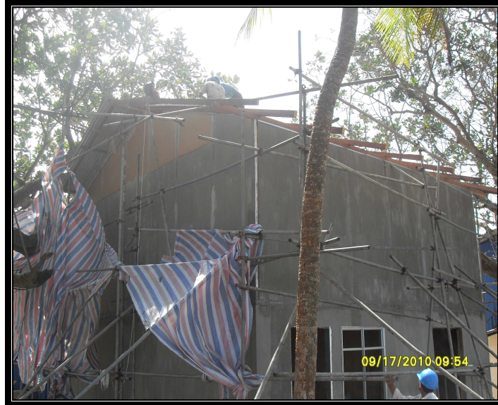
Figure 9: Side view of the two storey house under construction at Chaaya Bay hotel at Beruwala
