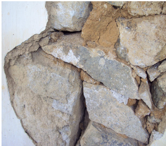
Fig 3.3 Rubble and clay mortar used to build walls in a bungalow at Hanthana, Kandy
