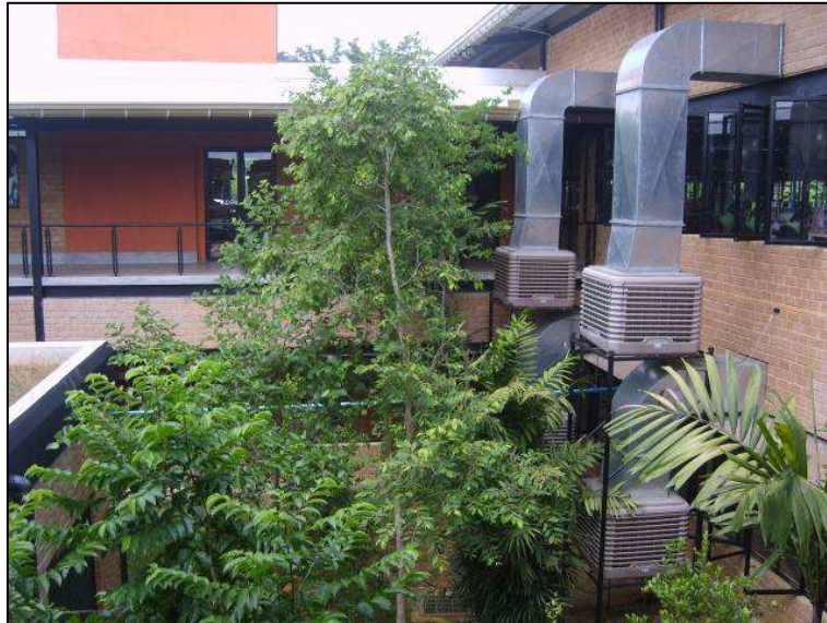
Figure 4: An evaporative cooler installed in a factory building
