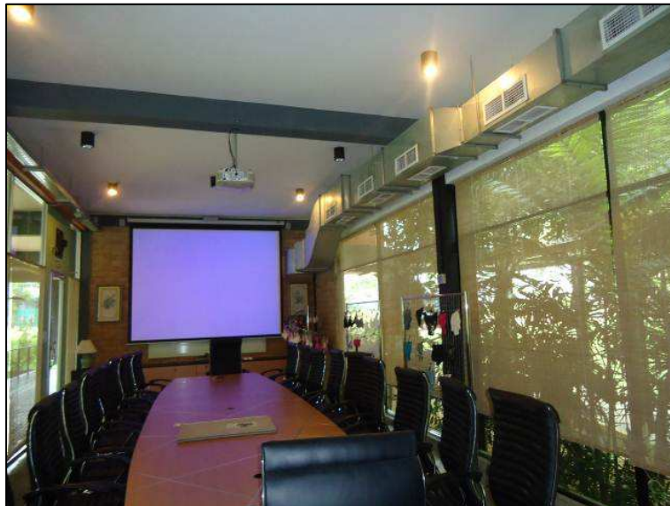
Figure 5: Conference room cooled by an evaporative cooling
