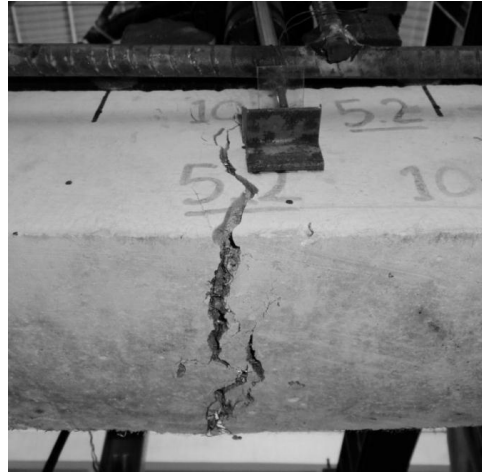
Fig.10: Growth of Crack pattern and failure of Micro-Fibers (i.e. Polymer fiber)
