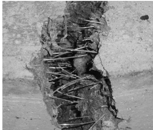
Fig.12: Zoomed view of pull out of Steel fibers after full development of crack
