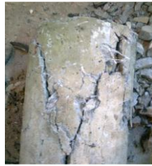
Figure 8: Wedge failure were observed in specimen C_2 and C_3
