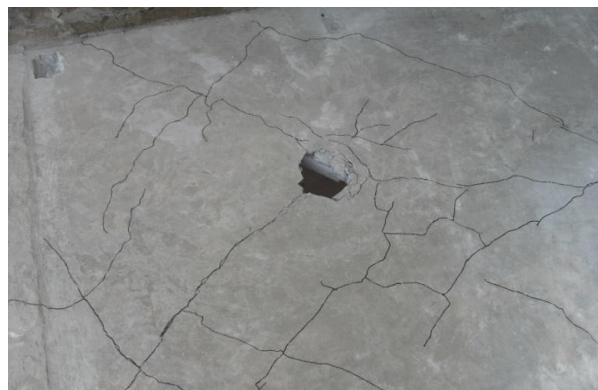
Figure 14: Crack at Point d
