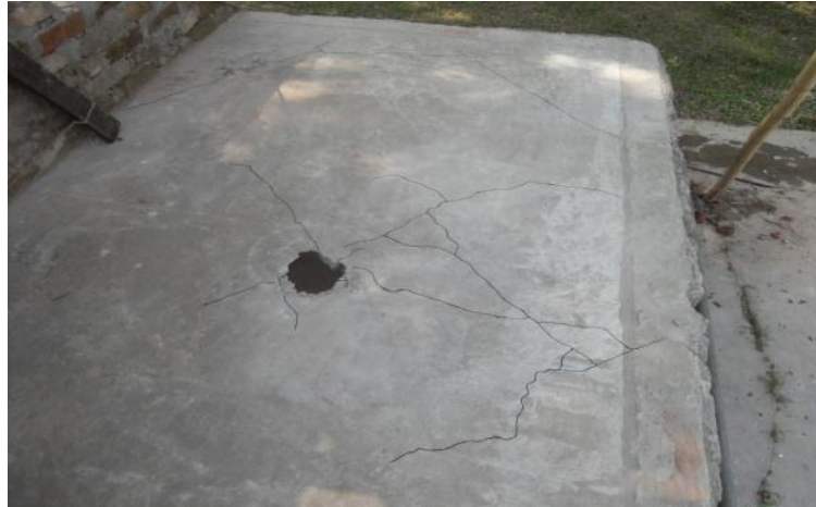
Figure 15: Crack at Point e
