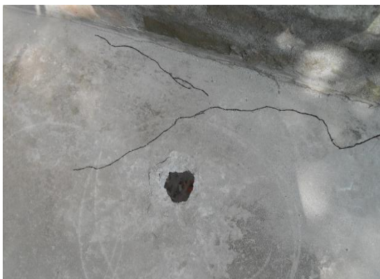
Figure 13: Crack at Point c
