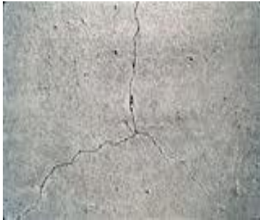
Figure 1: Plastic Shrinkage cracks in concrete structures
