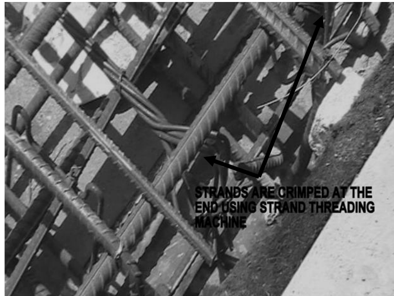
Figure 3: Practical usage of the Dead End Anchorage at site
