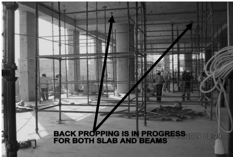
Figure 13: Back propping of the slab to do the slab casting above this level
