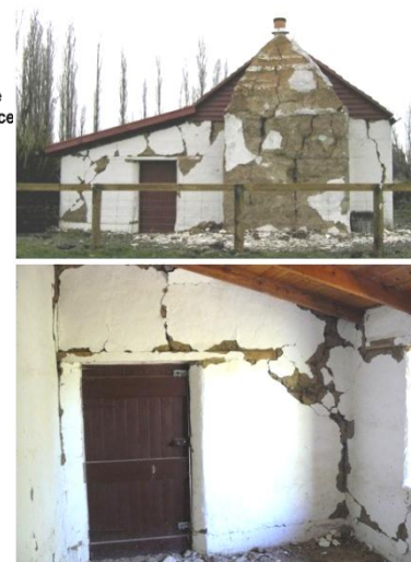
Figure 21 Cotons cob cottage extensively damaged
