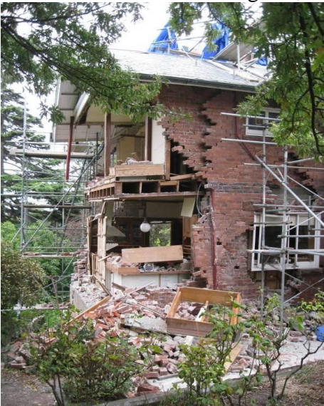
Figure 17 Examples of partial collapse of double brick houses (Carradine)
