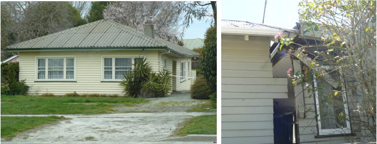
Figure 8 Houses near rivers that have been subject to differential settlement and lateral spreading
