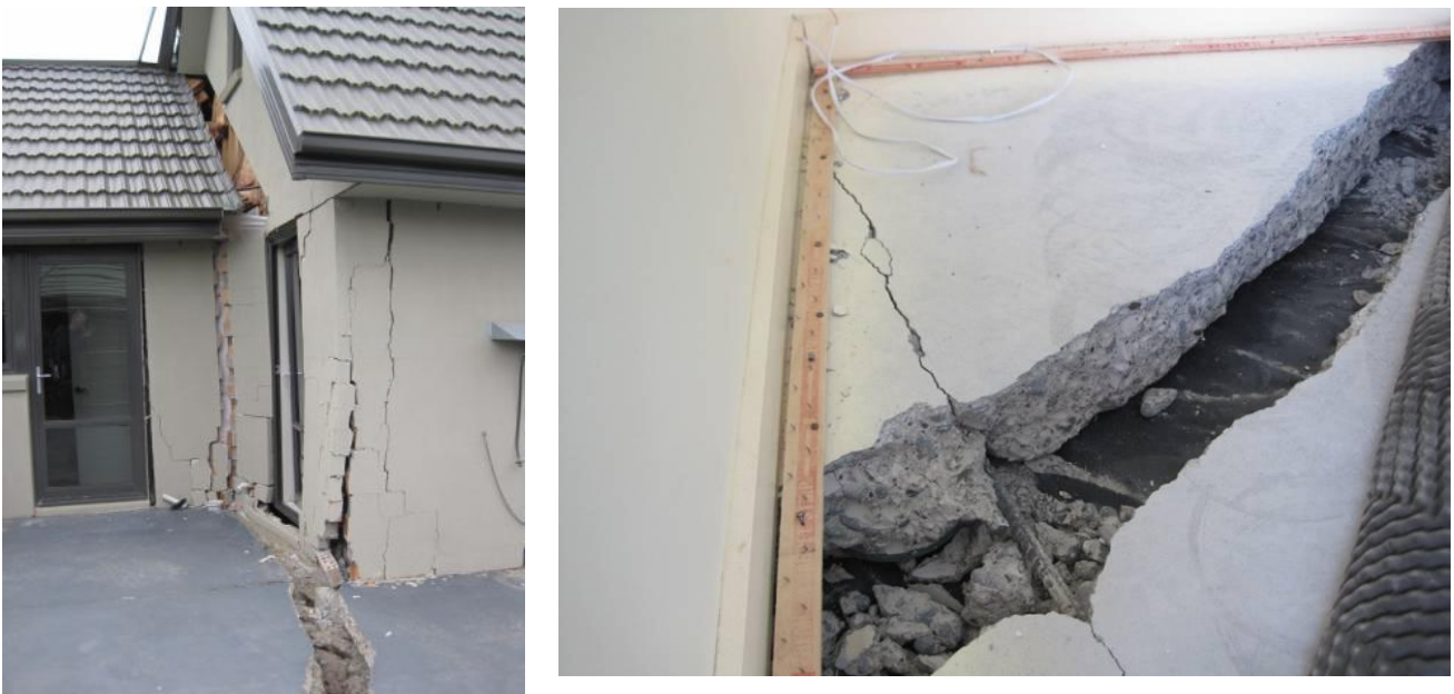
Figure 9 House and reinforced slab damage as a result of ground movement (Buchanan)
