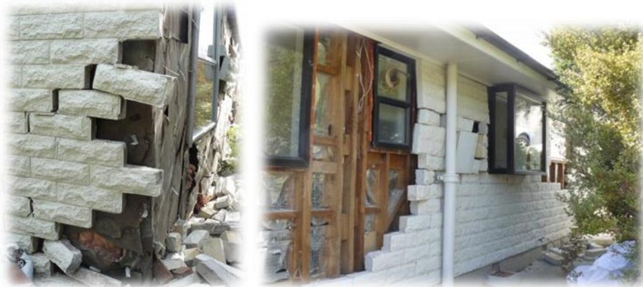
Figure 12 Two examples of masonry veneers detached from the wall framing. The first example with such poor mortar that the veneer has separated into individual bricks
