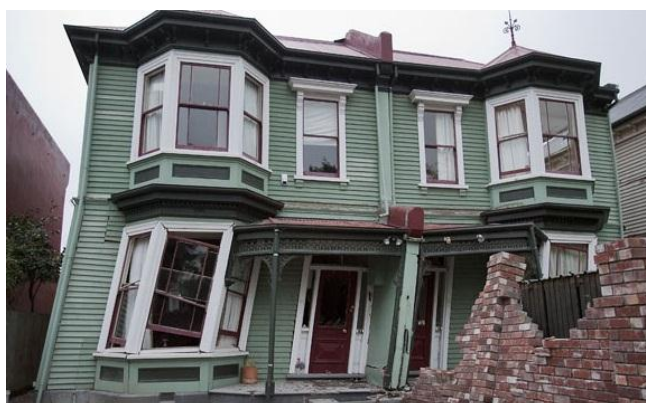
Figure 15. A soft storey failure of a timber framed house not resulting in collapse
