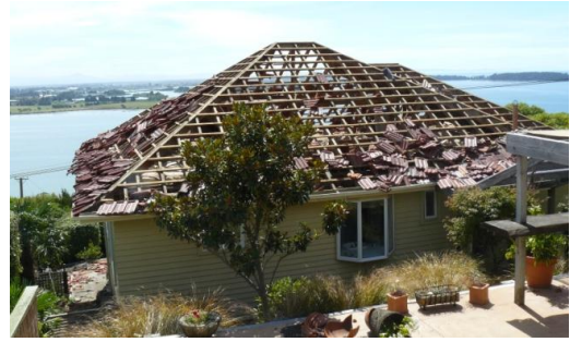
Figure 16 House with all roof tiles dislodged
