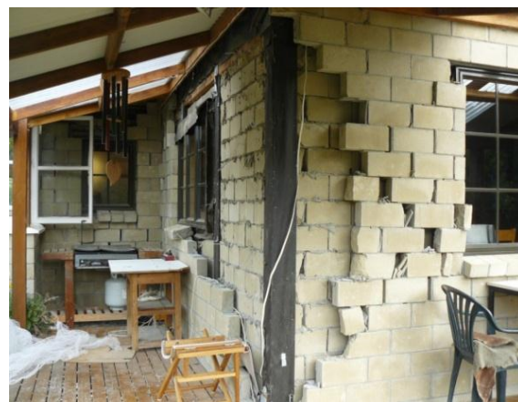
Figure 25 Pressed earth double skin masonry, serious wall failures were avoided because of the post and beam construction supporting the upper storey.
