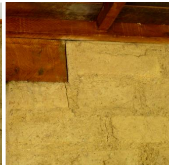
Figure 25 Opening at edge of lintel beam
