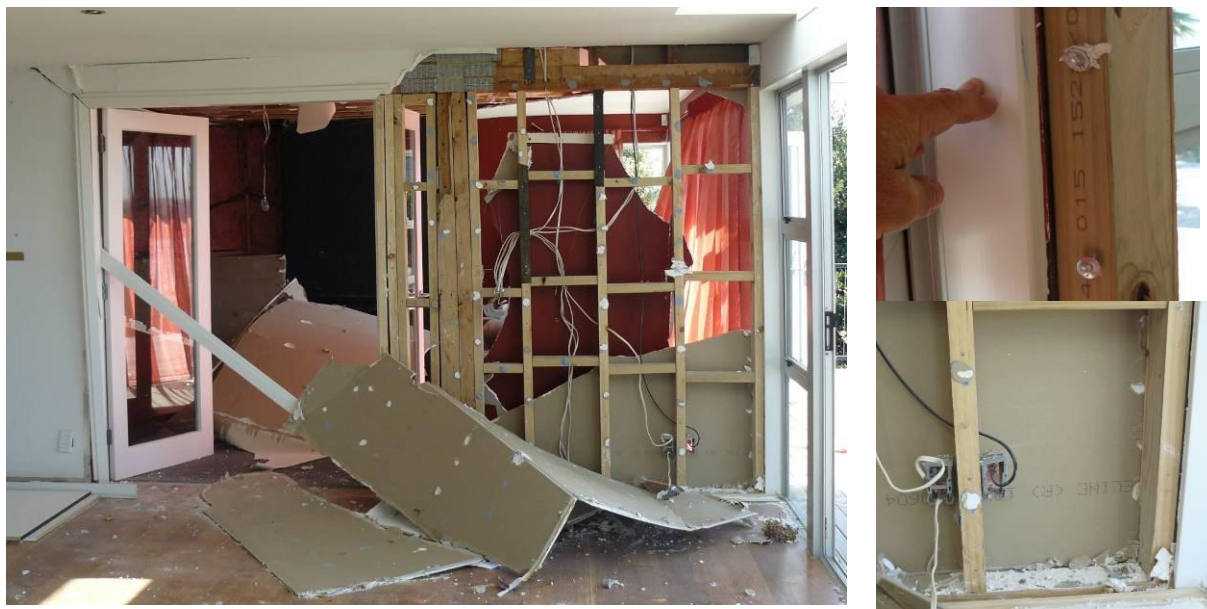
Figure 13. Severe failure of GIB Braceline internal linings (Morris)
