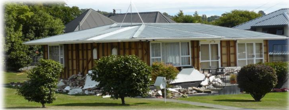
Figure 11 A house that totally lost its masonry and stucco facade
