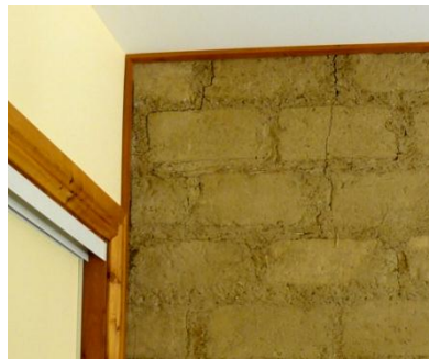
Figure 14 Crack in wall near the west corner
