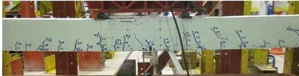
Figure 9: C50-SFARC-1.0% beam after failure
